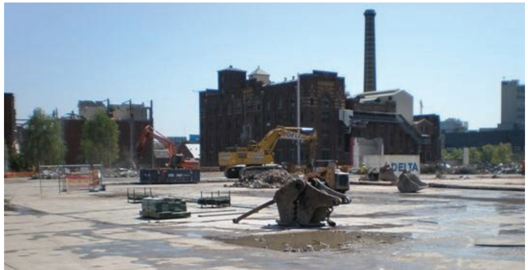
• Site clearing has nearly finished, this area will be transformed into the main park.
